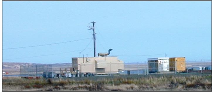
AVEC's new backup generator for St. Michael.
