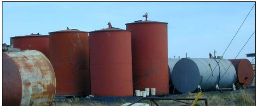
St. Michael Fuel Company’s bulk fuel tank farm located on the west side of the St. Michael.
