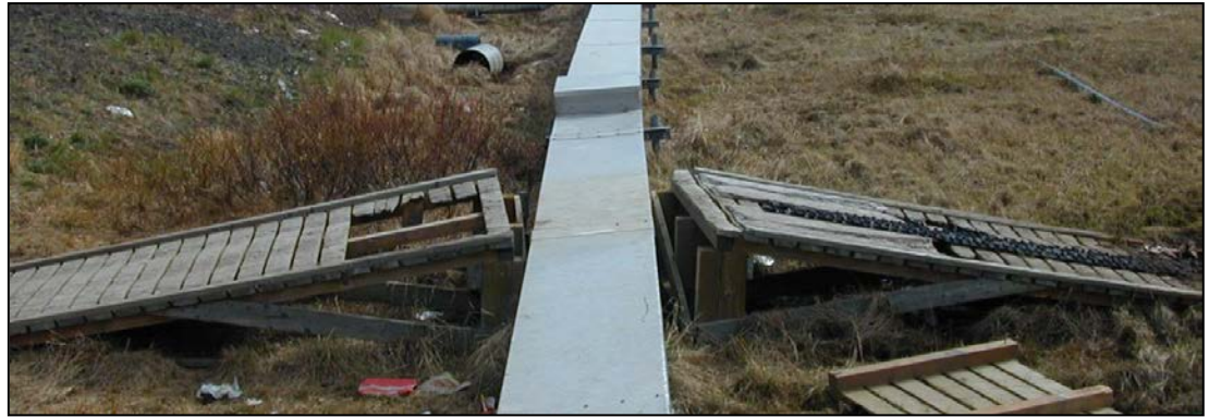
The above ground vacuum sewer system poses challenges for navigation and board walks and ramps need regular maintenance to insure safety.
