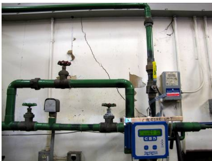
Walls of Water Plant are splitting from floor to ceiling.
