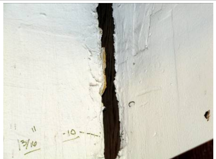
The walls in the Water Plant are splitting wide from floor to ceiling.
