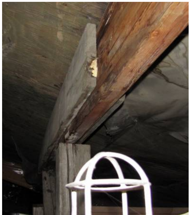
The main beam of the Water Plant is rotting, collapsing, and being held together by supports on both sides and below.
