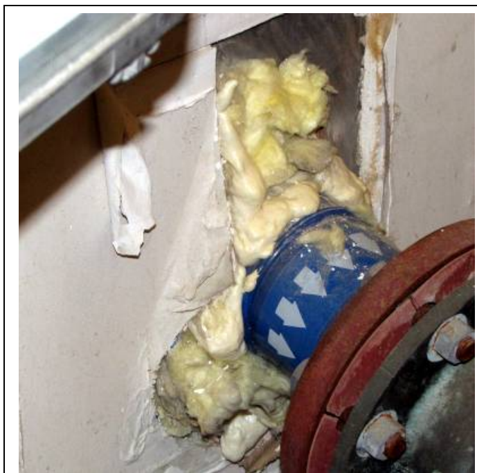
Sagging walls are cut to alleviate the pressure on the pipes in the water & sewer plant.
