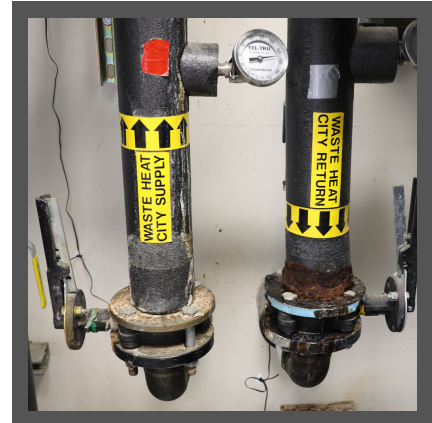
HEAT SUPPLY & RETURN - Waste heat from the City of Golovin power plant is supplied to the local washeteria. The loop returns back to the power plant and circulates to other facilities in the community. Photo by Kawerak, Inc.
