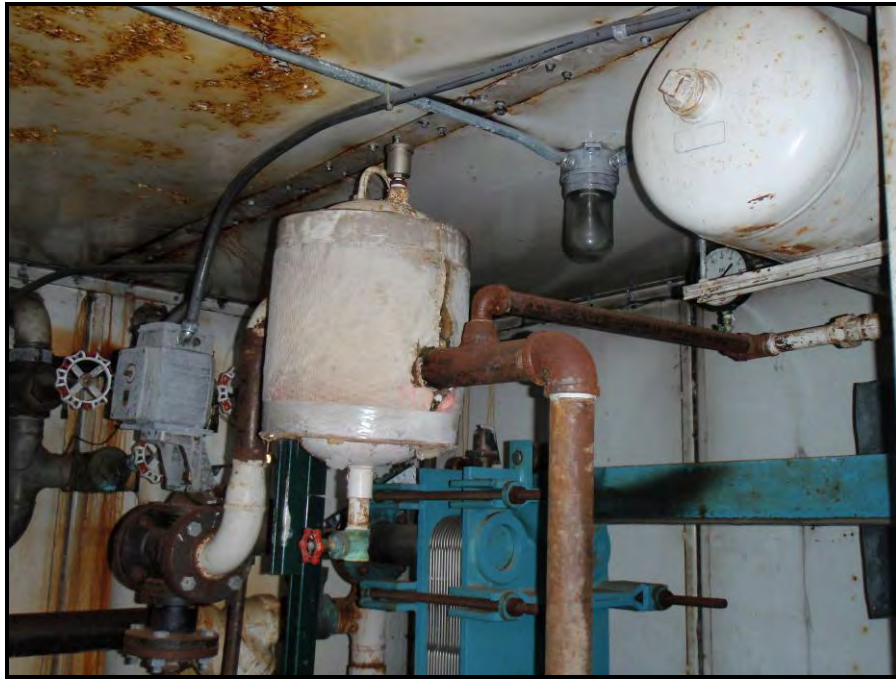
Photograph 11: Equipment remaining inside the white generator building.
