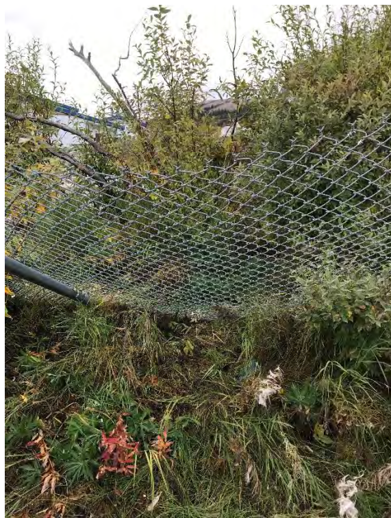
Photo 3: southwest fence collapsing into tank farm
