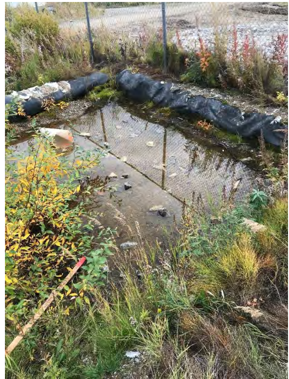
Photo 8: Standing water in southern portion of tank farm footprint
