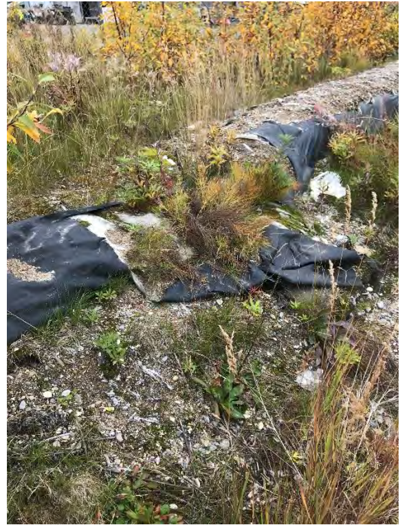
Photo 6: Tank farm berm condition
