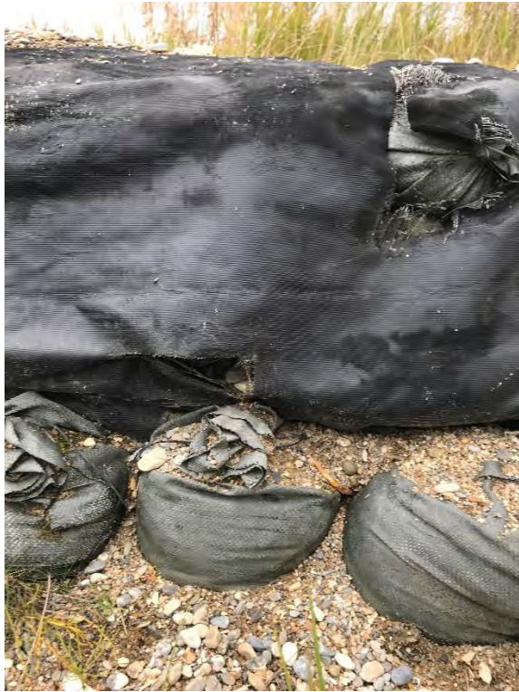
Photo 5: Tank farm berm condition
