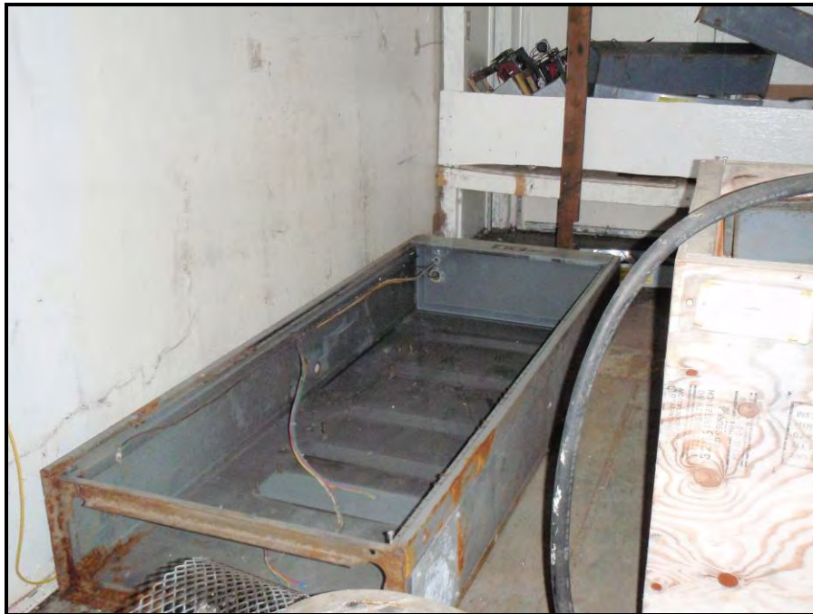
Photograph 14: Old generator base and electrical equipment present inside the CONEX building.
